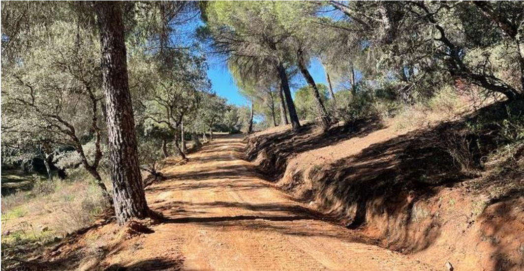
Figure 9: Country road improvement in La Tejera, Road surfacing can be easily compacted with a heavy beam. Ditches should be cleaned in the runoff areas near foci and/or heavily affected areas, channelling runoff to the main water courses.
